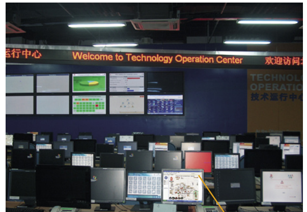
Technology operation center Beijing
